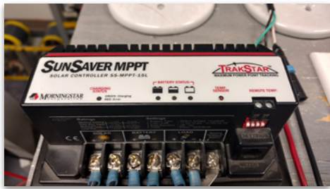
Figure 2.2.1: MPPT within panel not functioning
