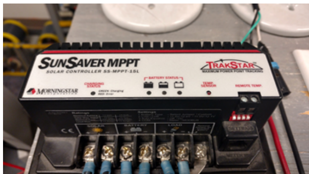
Figure 2.2.1: MPPT within panel not functioning
